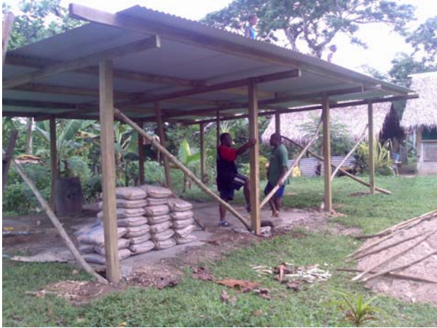
Shelter being built at Mango Station, Santo with materials provided by Canberra donations.
